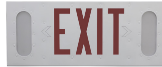
Exit Sign with Emergency Light
